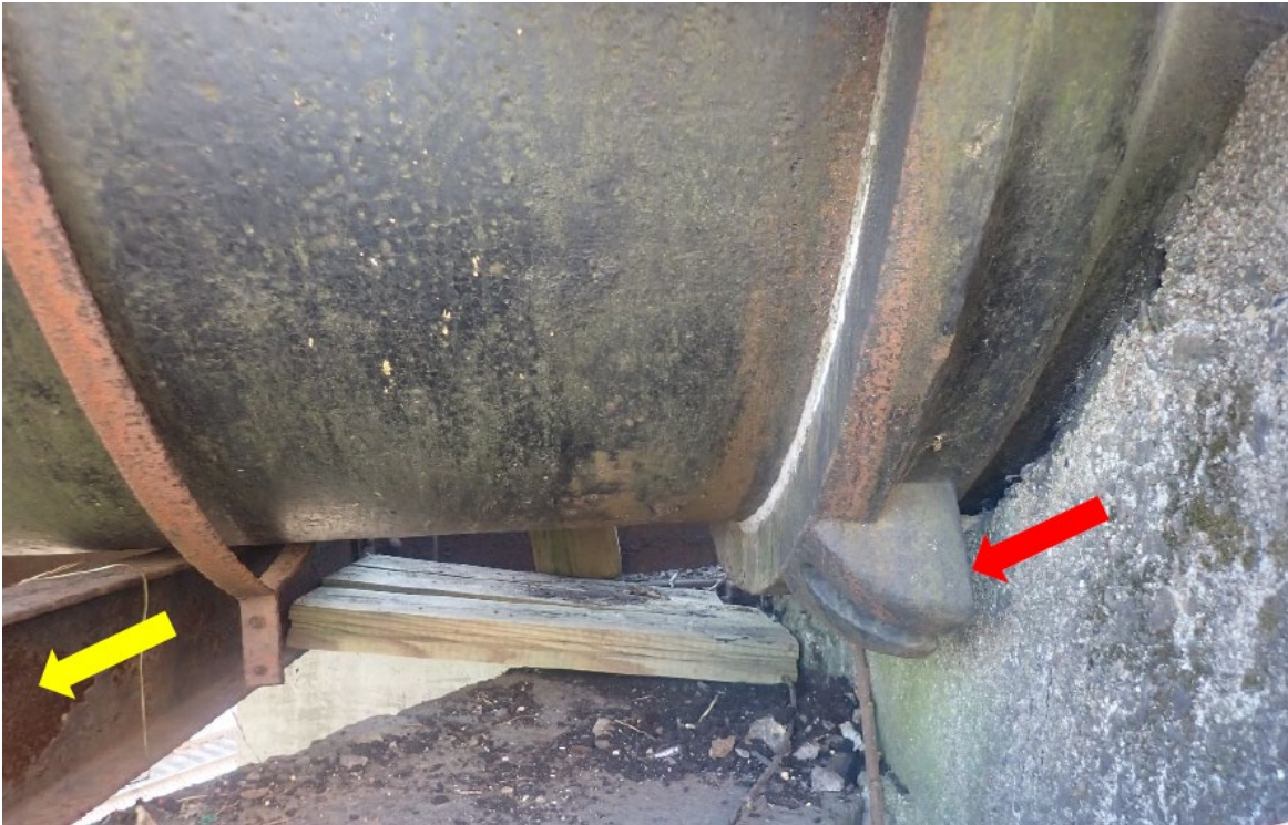
Attachment point for missing rod highlighted with red arrow. Obstructing structural member highlighted with yellow arrow.
